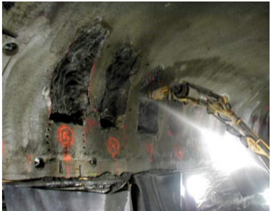
The Brokk machines were able to break concrete almost directly above their position
