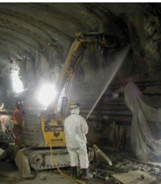
The compact size of the Brokk units made them the right fit in the narrow tunnels
